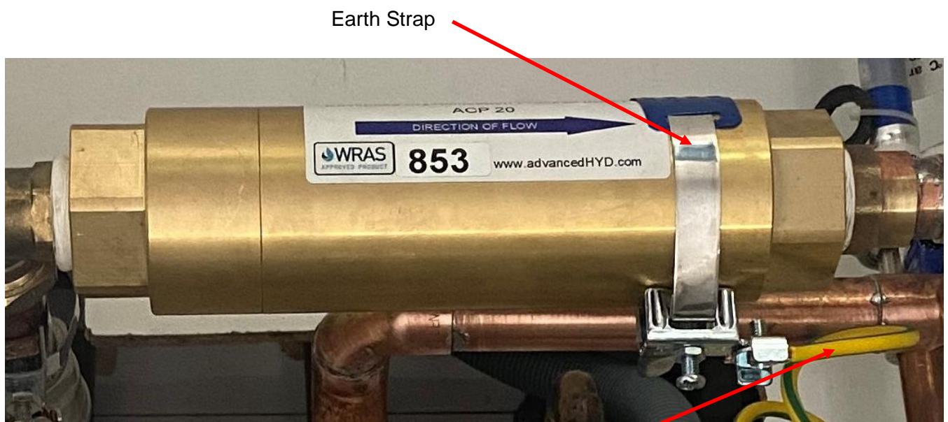
Earth lead connected to suitable earth point
